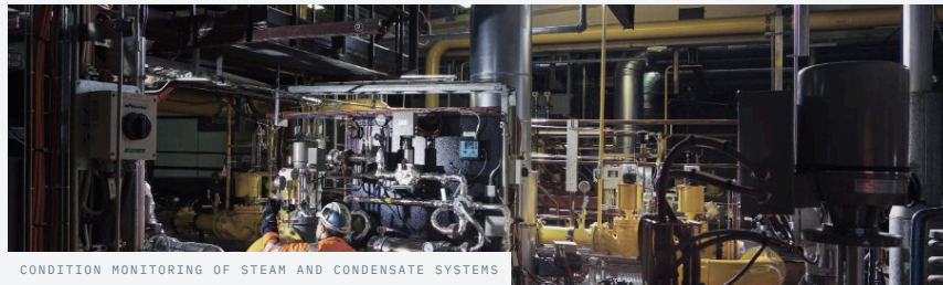
CONDITION MONITORING OF STEAM AND CONDENSATE SYSTEMS
